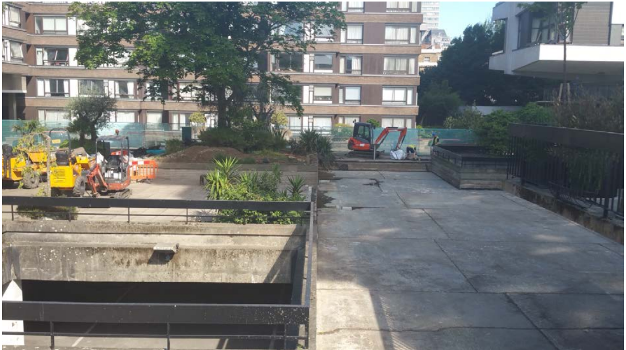
View of Water Gardens. Example of lightwell to be infilled to left.
